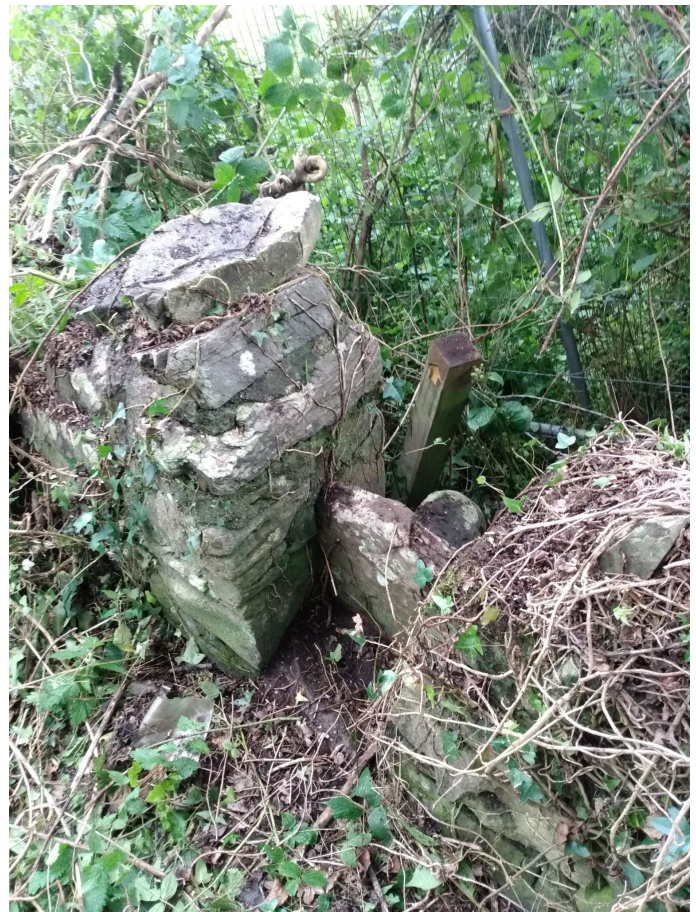
Photo 5 — Issue 5 as seen from above. Lecale Way marker post can be seen clearly. Heras fencing has been placed against the wall stopping use.
